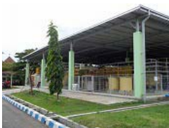
Wastewater treatment facility at YMPI
