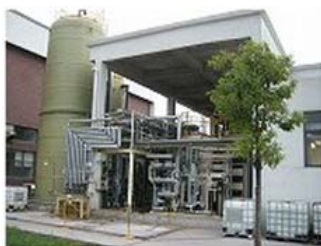
Wastewater treatment facility (Xiaoshan Yamaha)
