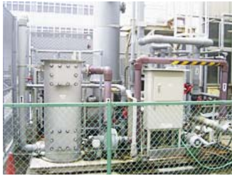
Groundwater purification equipment at the headquarters business site
