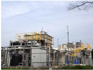
Wastewater treatment facility at the Kakegawa Factory
