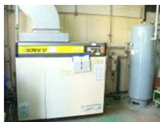
Compressor in which the pressure has been set at an appropriate level
