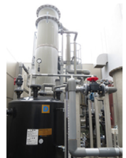
Groundwater purification equipment at our headquarters
