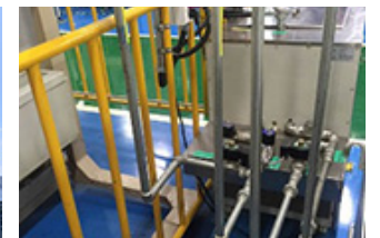
Cooling unit using circulated water
