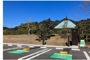
Electric vehicle charging stations that use renewable energy
