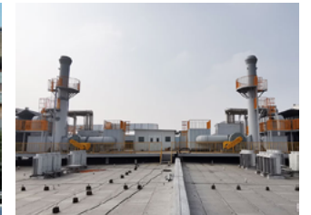
VOC treatment facility at Hangzhou Yamaha Musical Instruments Co., Ltd.
