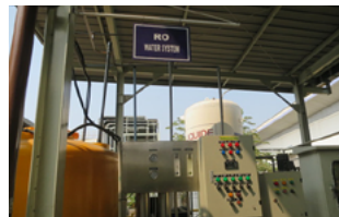
Reverse osmosis membrane equipment
