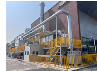
VOC treatment facility at Xiaoshan Yamaha Musical Instruments Co., Ltd.
