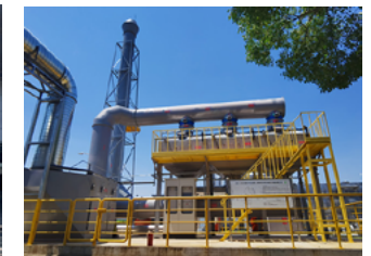
VOC treatment facility at Yamaha Electronics (Suzhou) Co., Ltd.
