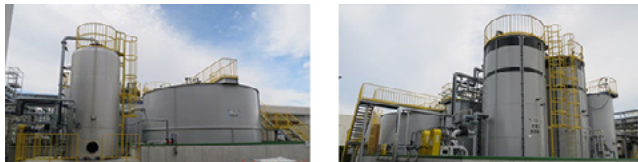
Wastewater processing equipment at the main factory of Yamaha Music Manufacturing Japan
