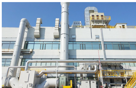
VOC treatment facility at Hangzhou Yamaha Musical Instruments Co., Ltd.
