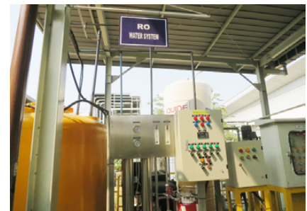
Reverse osmosis membrane equipment
