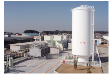
Cogeneration system at Kakegawa Factory
