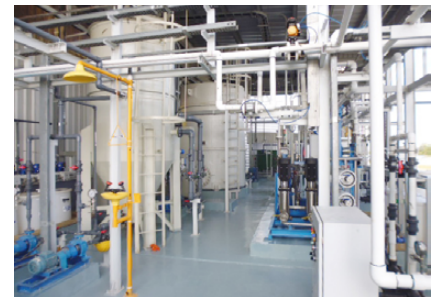
Reuse of 100% of manufacturing process wastewater
