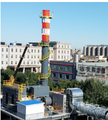
VOC treatment facility at Tianjin Yamaha Electronic Musical Instruments, Inc.
