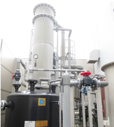
Groundwater purification equipment at our headquarters
