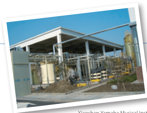
Xiaoshan Yamaha Musical Instrument Co., Ltd. The cutting-edge wastewater treatment plant
