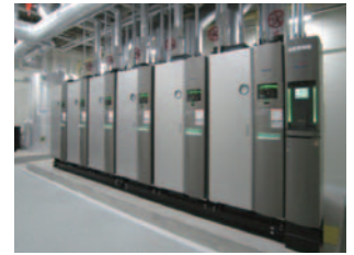
The natural-gas-fired boiler
