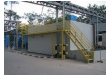
Wastewater treatment system at YMMI
