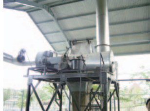
The YMPI sludge dryer
