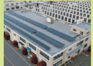
Photovoltaic Power Generation System (Factory at Yamaha headquarters)
