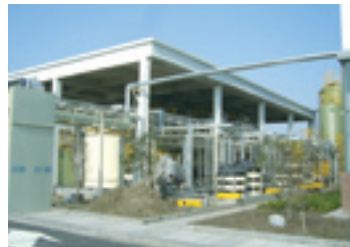
State-of-the-art wastewater treatment facility installed in production process in new Xiaoshan Factory, China
