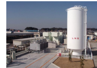
Cogeneration system at Kakegawa Factory
