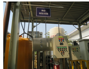
Reverse osmosis membrane equipment
