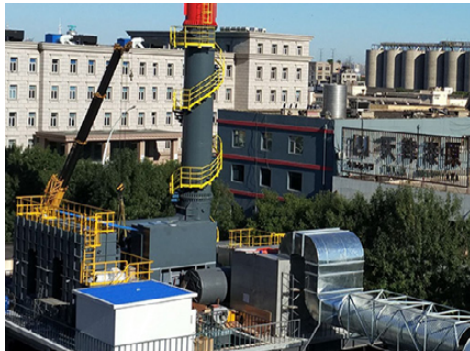
VOC treatment facility at Tianjin Yamaha Electronic Musical Instruments, Inc.
