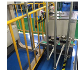
Cooling unit using circulated water
