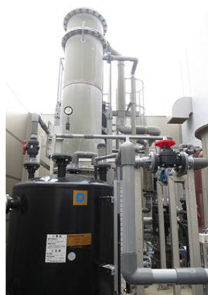
Groundwater purification equipment at our headquarters
