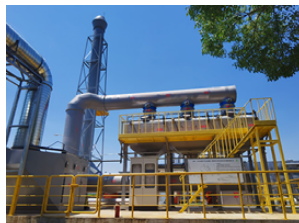
VOC treatment facility at Yamaha Electronics (Suzhou) Co., Ltd.
