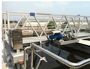
Reuse of wastewater for cooling water
