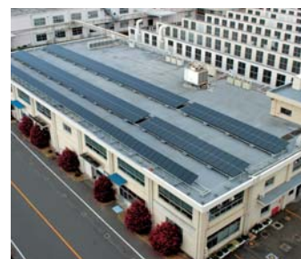
Photovoltaic power generating system
