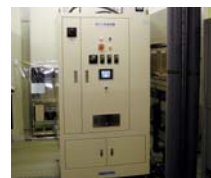
Exhaust gas treatment system (Yamaha Kagoshima Semiconductor Inc.)
