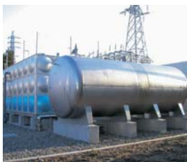
Well water tank (Toyooka Factory of Yamaha Corporation)
