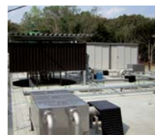
Enhanced septic tank
