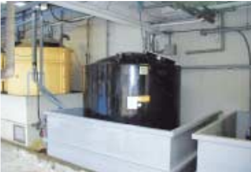
Fluid-retention barrier at the wastewater treatment facility in the Saitama Factory
