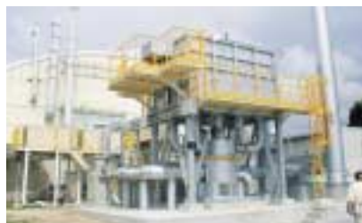
Regenerative exhaust-gas heat treatment system (Tenryu Factory)
