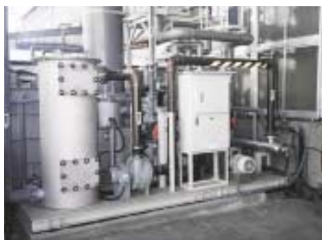
Remediation facilities (Main Factory)
